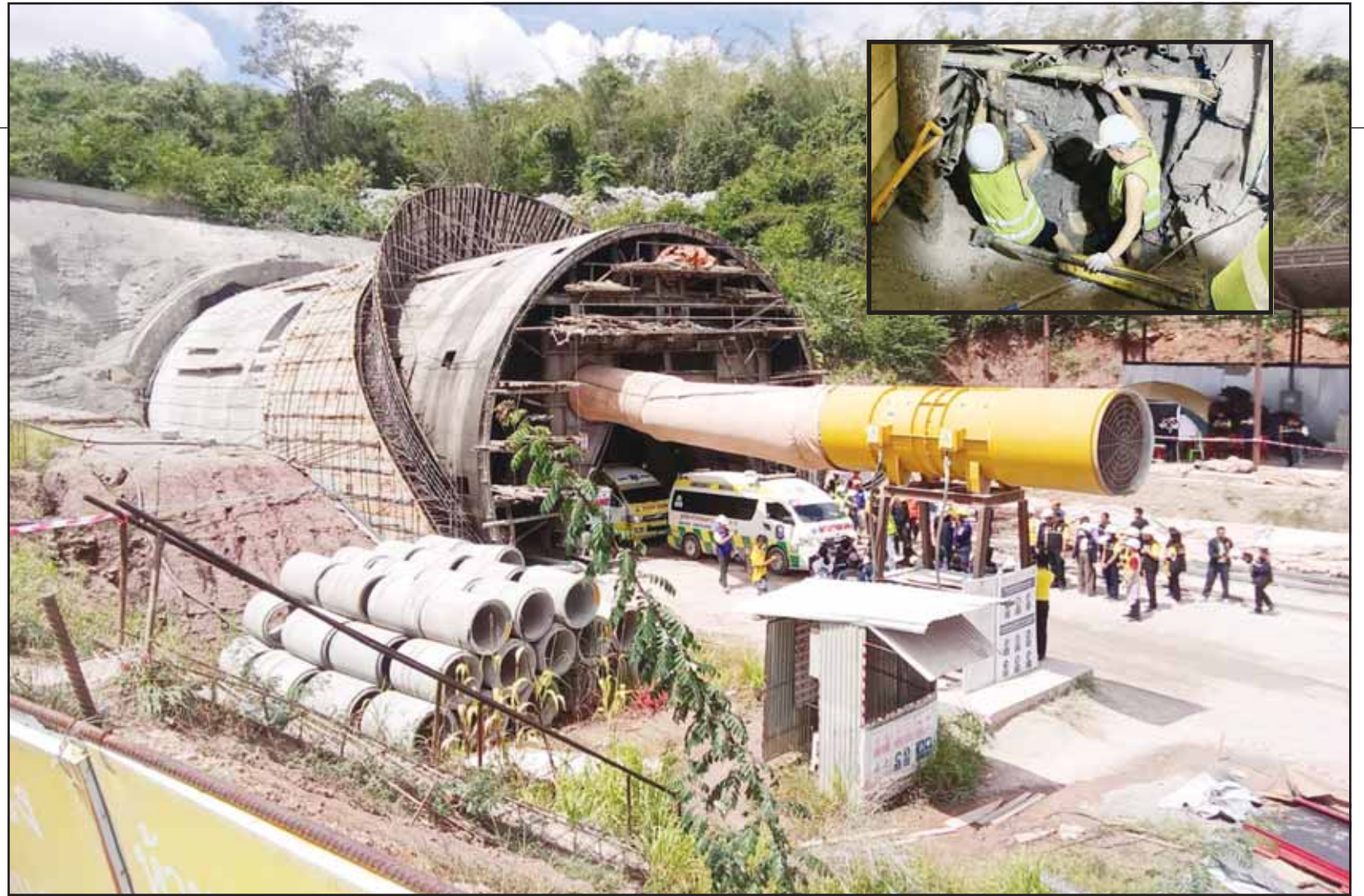
In this photo released by the State Railway of Thailand, ambulances are prepared on Aug 30, to carry away bodies of two workers who had been trapped in a collapsed tunnel in Nakhon Ratchasima province, Thailand, that is part of the Thai-Chinese high-speed railway construction site. Inset: In this photo released by the State Railway of Thailand, rescuers work on Aug 29 at the scene of a collapsed tunnel in Nakhon Ratchasima province that is part of the Thai-Chinese high-speed railway construction site. (AP)
