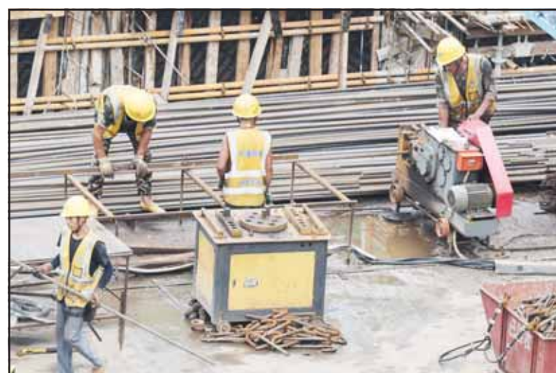
Workers work at a construction site in Haikou, south China's Hainan Province on Sept 11. Hainan has witnessed its production gradually resumed after Super Typhoon Yagi, the 11th typhoon of the year, made landfall in Hainan on Friday and brought damage across the island. (Xinhua)
