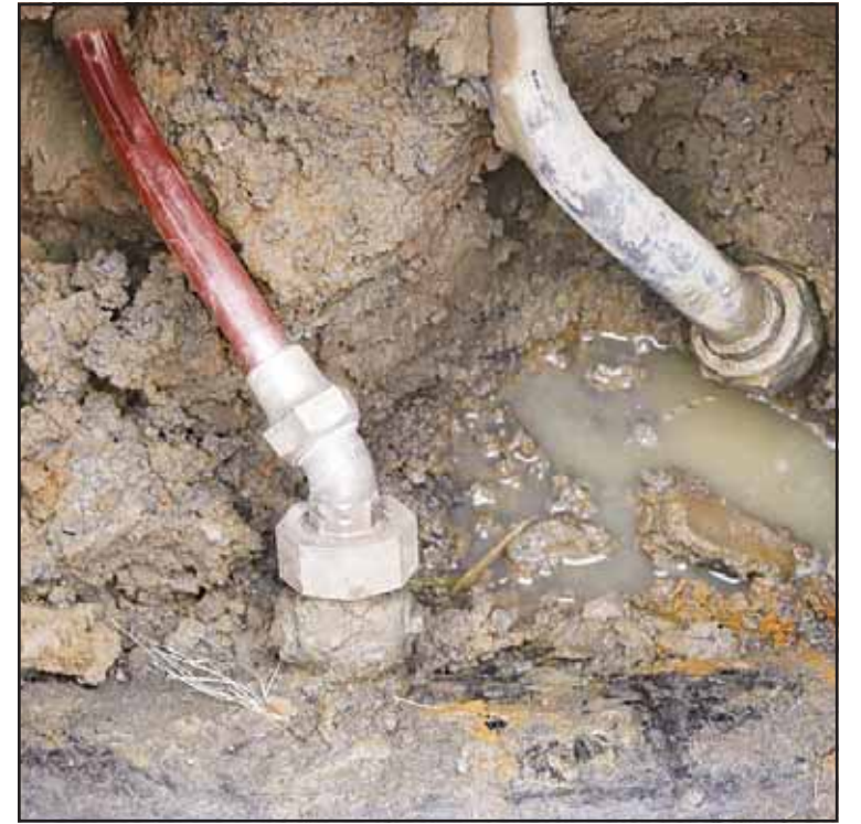
A copper water supply line (left), is shown connected to a water main after being installed for lead pipe (right) on July 20, 2018, in Flint Michigan. (AP)
