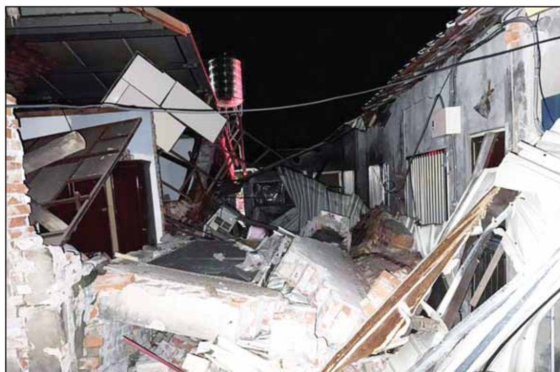
This photo taken on Jan 21, 2025 shows damaged buildings after an earthquake in Tainan City, southeast China's Taiwan. (Xinhua)
