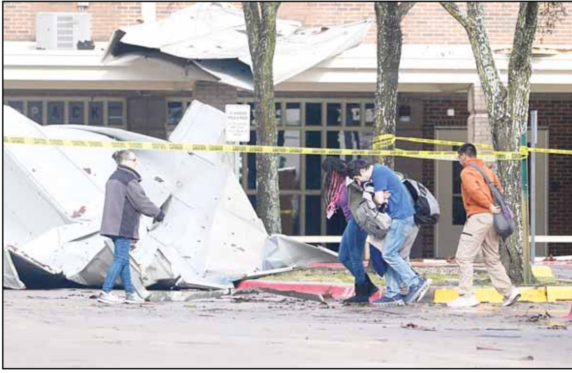
Students arriving for classes walk past damage from the roof that was sheered off by high winds at Plano West High School on March 4 in Plano, Texas. (AP)
