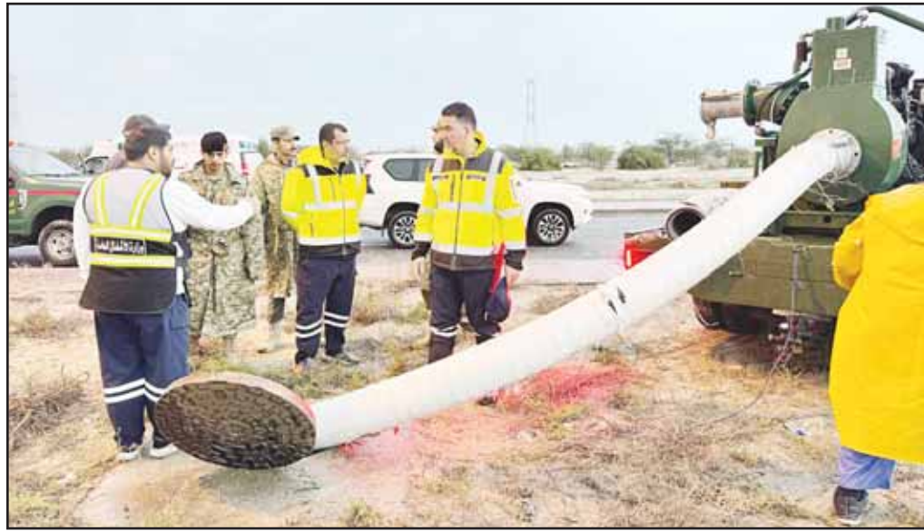
National Guard Fire Department emergency teams provide support to the Ministry of Public Works and the General Fire Force in dealing with water pools.
