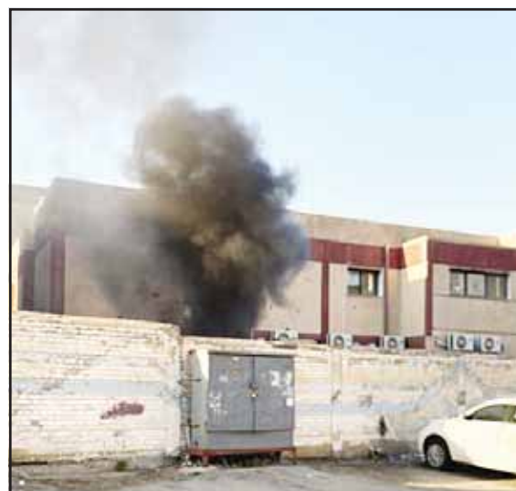
Smoke billows from power transformer.
