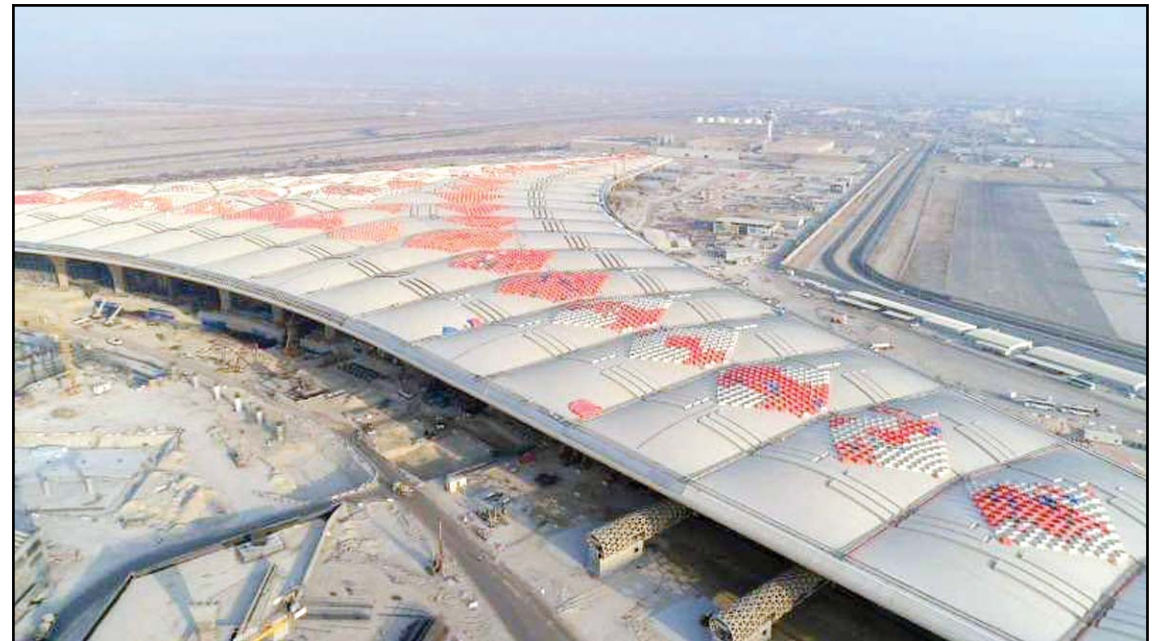
Aerial shot of the ongoing construction of the new passenger terminal at Kuwait International Airport.
