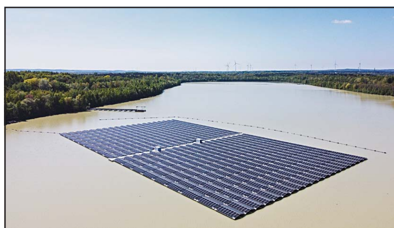
Solar panels on Germany's biggest floating photovoltaic plant produce energy under a blue sky on a lake in Haltern, Germany, on May 3. Germany's energy minister announced plans Friday, May 5, to ease bureaucratic hurdles for solar power as the country set a new record for photovoltaic installations during the first quarter. Europe's biggest economy added 2.7 Gigawatts of solar power capacity during the first three months of 2023, putting it on course to beat the target of 9 GW this year, up from 7 GW in 2022. (AP)
