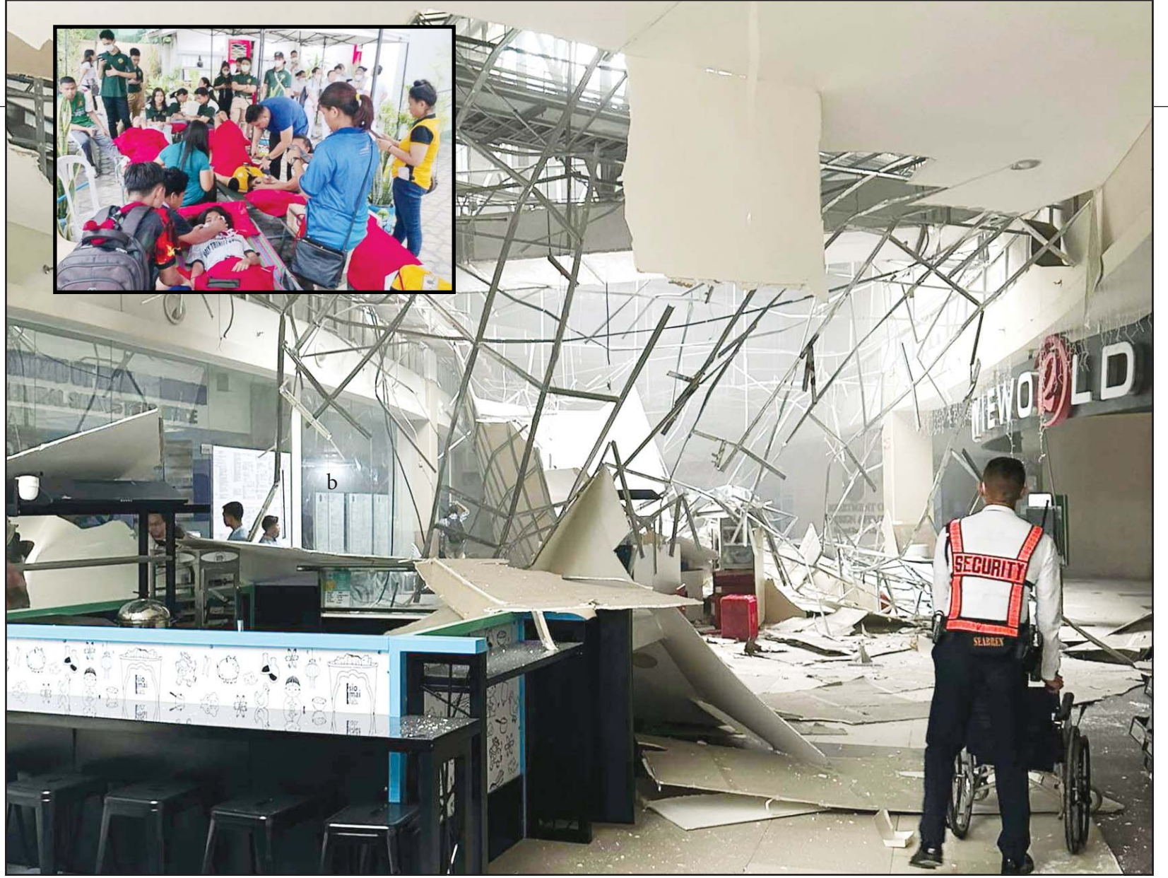
A security guard walks beside the damaged ceiling of a shopping mall in General Santos City, South Cotabato, southern Philippines on Nov 17. A powerful undersea earthquake has shaken the southern Philippines. The US Geological Survey says the quake measured magnitude 6.7 and was located 26 kilometers
