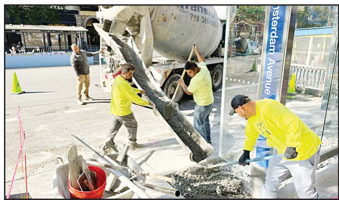
Workers pour concrete to create part of a bus stop in the Manhattan borough of New York City on Thursday, October 12, 2023. On Friday, the U.S. government issued the October jobs report. (AP)
