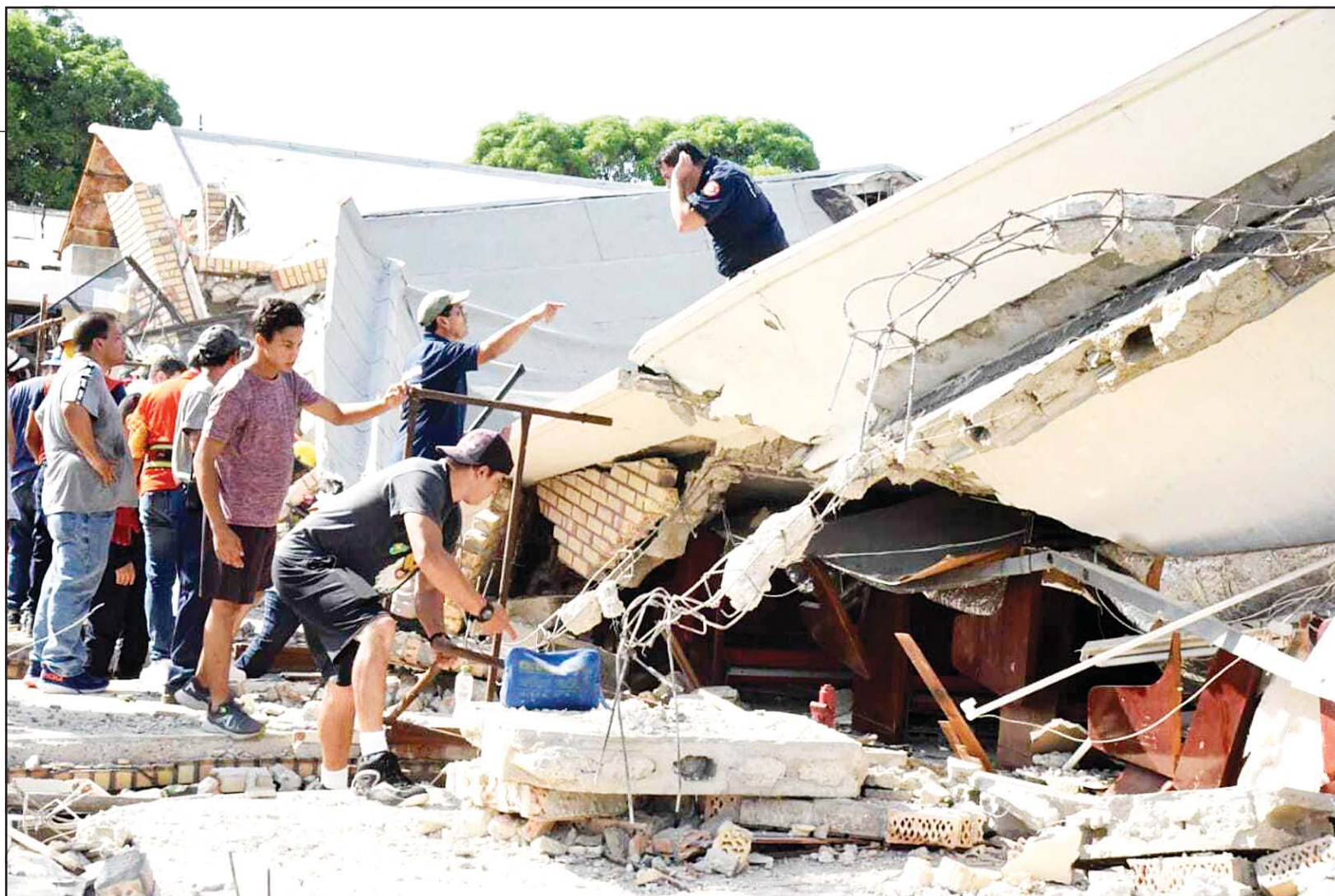
Rescue workers search for survivors amid debris after the roof of a church collapsed during a Sunday Mass in Ciudad Madero, Mexico on Oct 1. The Bishop of the Roman Catholic Diocese of Tampico said the roof caved in while parishioners were receiving communion. (AP)
