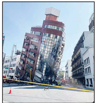
In this photo released by the Hualien City Government, a leaning building is cordoned off in the aftermath of an earthquake in Hualien, eastern Taiwan on April 3, 2024. (AP)
