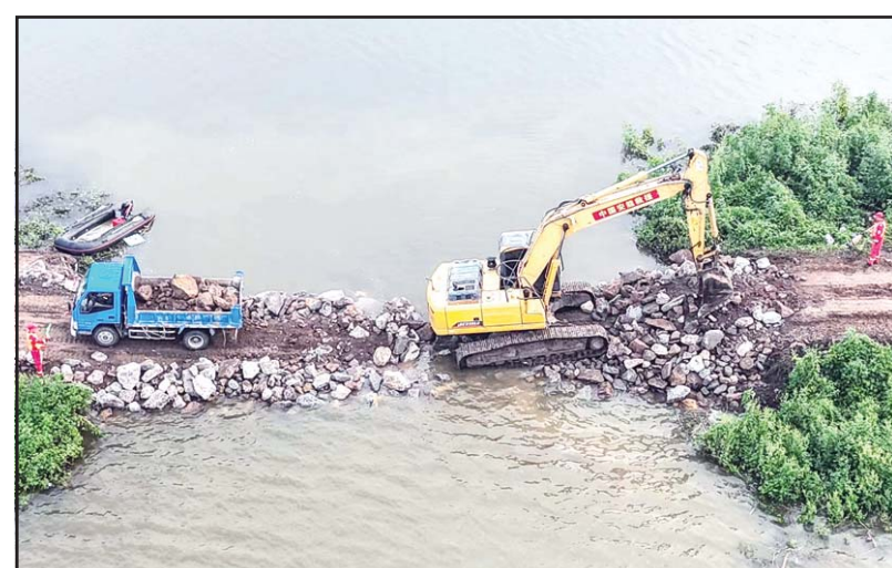
This aerial drone photo taken on Aug 7, 2024 shows emergency workers attempting to seal a dike breach in Tieling, northeast China's Liaoning Province. The dike breach at a river in northeast China's Liaoning Province was sealed at 4:27 am on Wednesday after emergency workers had worked around the clock to repair it, according to local authorities. (Xinhua)
