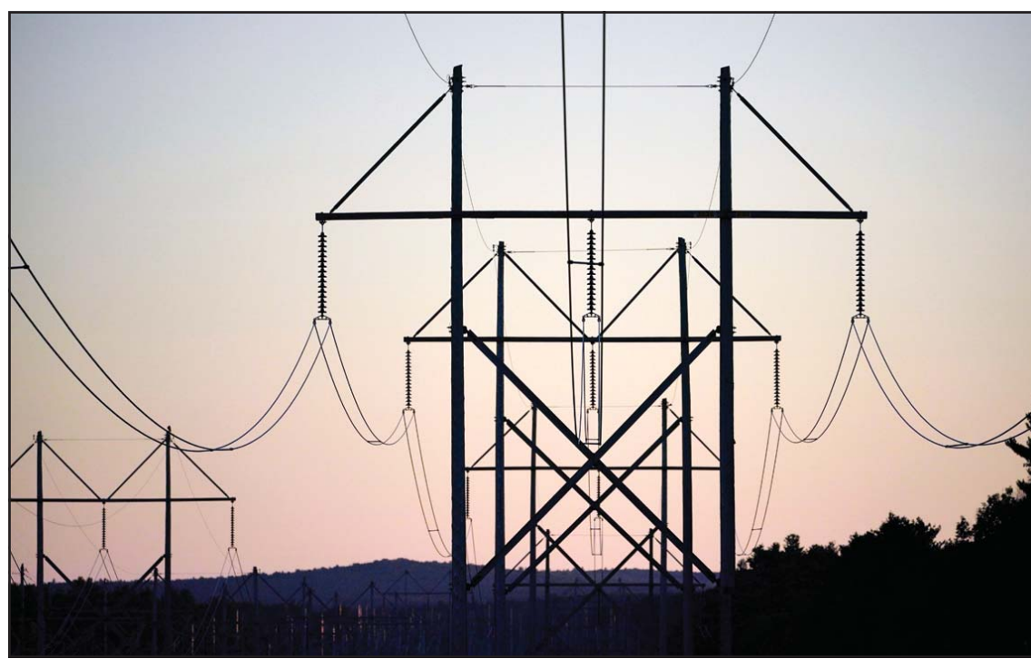
Central Maine Power transmission lines stretch above the treetops in Pownal, Maine, on Oct. 6, 2021. (AP)
