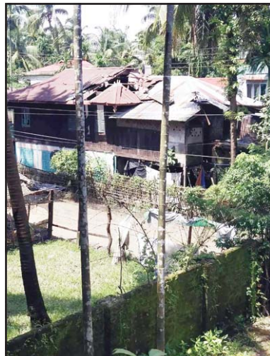
A view of the roof of a house damaged by bombs dropped from a drone in Ali village in Maungdaw township, Rakhine state, Myanmar on Aug 10. (AP)
