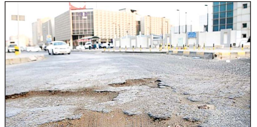
Broken roads with potholes can cause serious accidents.
