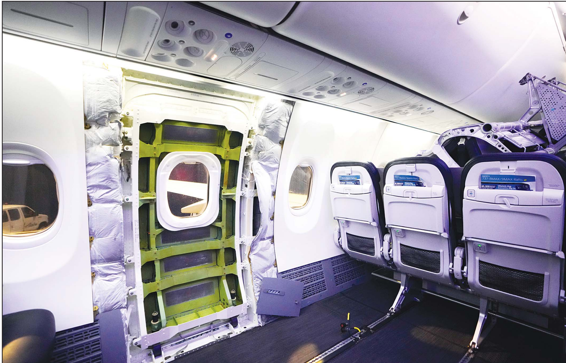
A door plug area of an Alaska Airlines Boeing 737 Max 9 aircraft awaiting inspection is pictured with paneling removed at the airline's facilities at Seattle-Tacoma International Airport Wednesday, Jan. 10, 2024, in SeaTac, Wash. The Federal Aviation Administration says it will audit Boeing's aircraft production and increase oversight of the troubled company after a panel blew off a jetliner in midflight last week. (AP)
