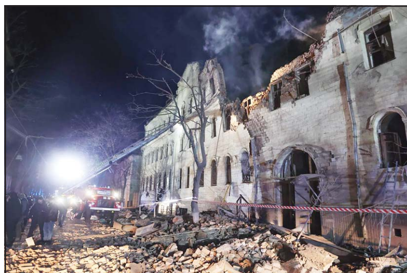
In this photo provided by the Kharkiv Regional Administration, an apartment building damaged in a Russian rocket attack is seen in Kharkiv, Ukraine, in the early hours of Jan 17. Russia fired two missiles during the night, hitting apartment buildings and a medical center and injuring 17 people, officials said Wednesday, in Moscow's latest strikes on civilian areas in the almost two-year war. (AP)
