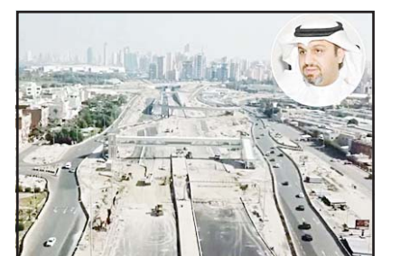
Aerial view of Cairo Street development project. Inset: Eng. Ahmed Al-Saleh, the official spokesman for the Ministry of Public Works and the Public Authority for Roads and Land Transport.
