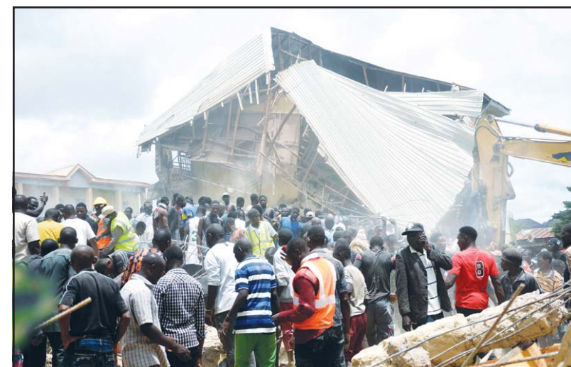
People and rescuers gather at the scene of a collapsed two-storey building in Jos, Nigeria, Friday, July 12. The school collapsed during morning classes on Friday in north-central Nigeria, killing 22 students and sending rescuers on a frantic search for more than 100 people trapped in the rubble, authorities said. (AP)
