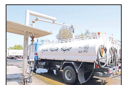
Fresh water filling station.
