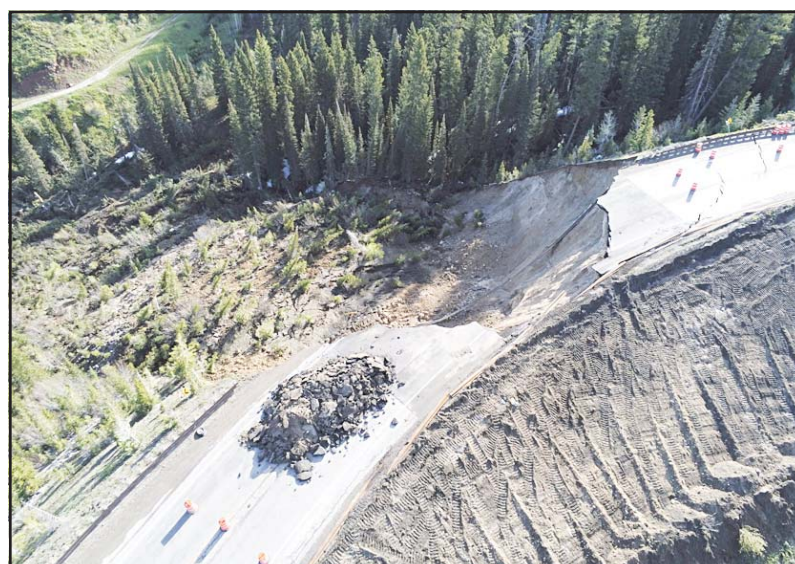
This photo provided by Wyoming Highway Patrol shows a damaged section of Teton Pass near Jackson, Wyoming on June 8 that officials said had 'catastrophically failed.' Aerial photos and drone video of the collapse show the Teton Pass road riven with deep cracks, and a big section of the pavement disappeared altogether. The road was closed at the time of the collapse. (AP)
