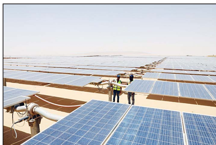
Workers check solar panels at the Benban Solar Energy Park in Aswan, Egypt, on April 21, 2024. Located in the desert of Aswan, a southern province of Egypt, the park covers an area of 37 square km and is planned to have a total installed capacity of two gigawatts. (Xinhua/Ahmed Gomaa)
