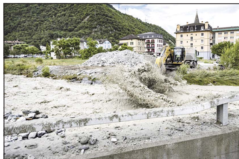
An excavator removes stones from the bed of the Navizence river, which flows into the Rhine, in Chippis, canton Valais, Switzerland on June 22. Three people were missing on Saturday after massive thunderstorms and rainfall in southeastern Switzerland caused a landslide, authorities said. (AP)
