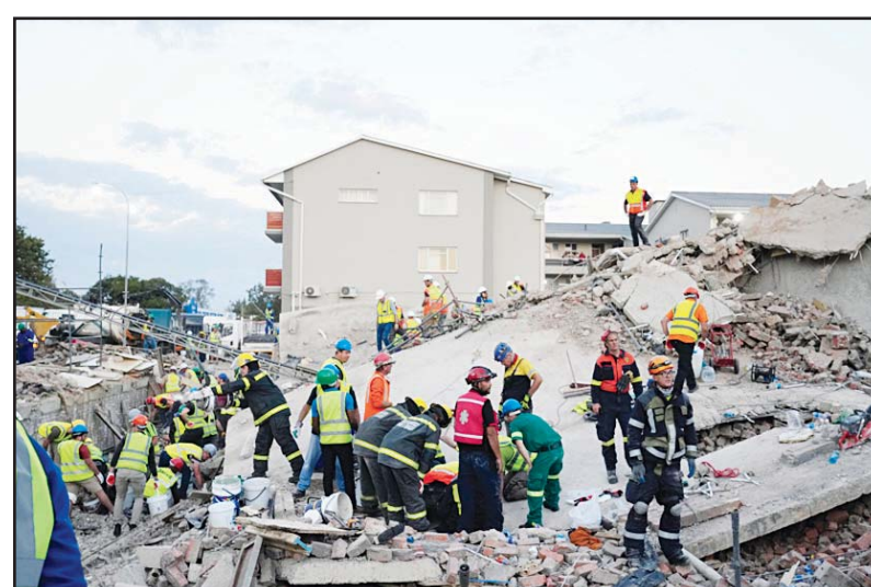
Emergency workers on the scene of a building collapse in the city of George, about 400 kilometers (250 miles) east of Cape Town, South Africa on May 7. An exhaustive rescue operation to find missing construction workers trapped in the rubble of a collapsed building in South Africa ended on May 17 after nearly two weeks, as authorities released a major revision of their figures and said they now believe that no one else is missing. (AP)
