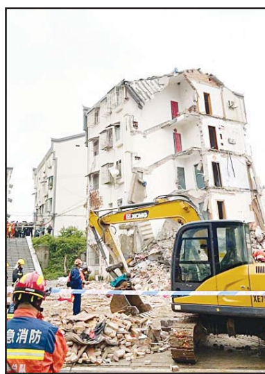
This photo taken on May 27, 2024 shows a collapsed residential building in Datong Township of Tongling City, east China's Anhui Province. A residential building partially collapsed on Monday afternoon in Datong Township of Tongling City, east China's Anhui Province, according to local authorities. The collapse occurred at around 1:40 pm. Rescue efforts are underway. (Xinhua)
